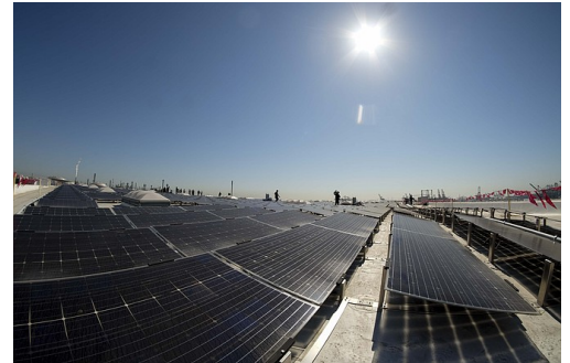
L.A. solar developer PermaCity Inc. has completed the world's most powerful solar rooftop generating project in San Pedro. Photo by Ringo H.W. Chiu
